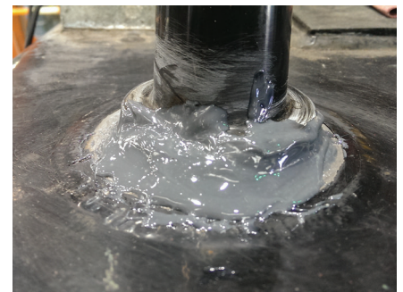
Sealed bushing leak
