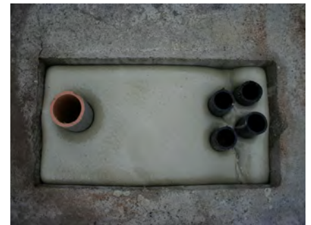
Completed installation in transformer pad
