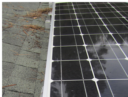
Clean panels maximize power production
